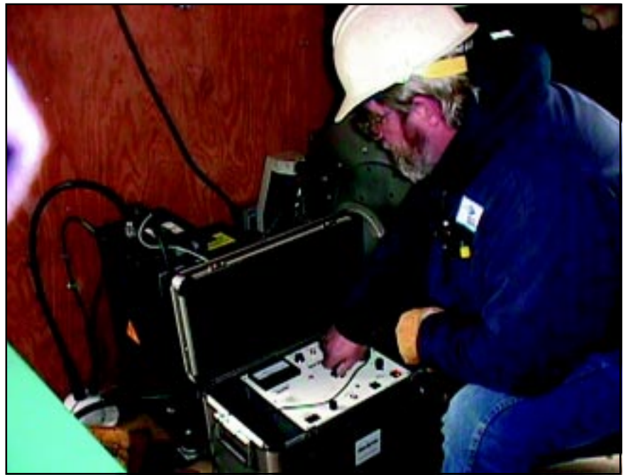
Fig. 1. Vaughn Reigner, PECO Energy electric operations foreman, adjusts the equipment for a cable test. A high-voltage tank is in the background.
